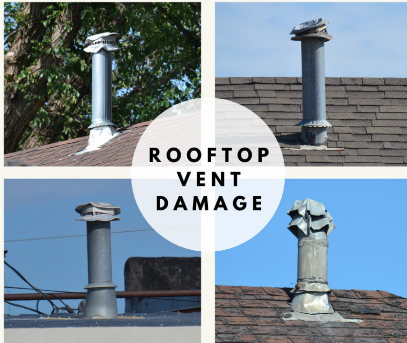
Damaged or covered gas exhaust vents prevent carbon monoxide (CO) from properly venting, and can lead to a deadly buildup of CO inside the home. CO is colorless and odorless, and only a carbon monoxide detector can alert homeowners to its presence. The Centers for Disease Control estimates 400 Americans die in their homes from unintentional CO exposure. The images above were taken after hail storms in Sheridan County in June 2024.
